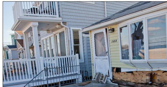
Thousands of dollars in flood damage can be prevented by building higher.
