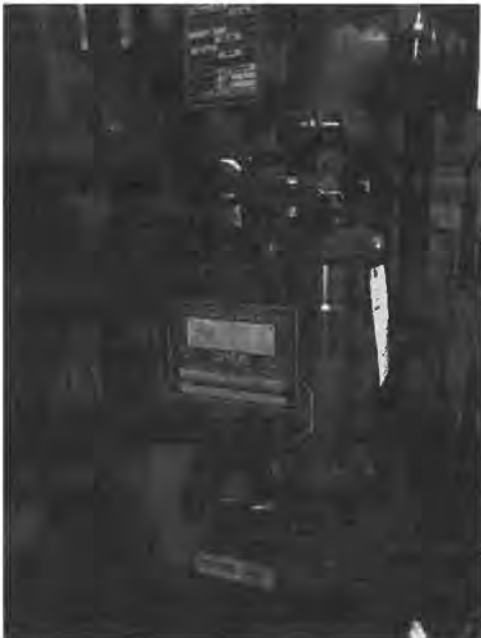
Sprinkler System Riser
